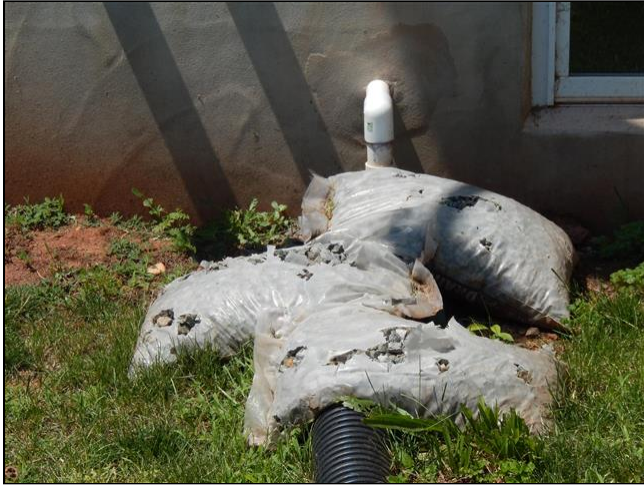
5.6 Item 2(Picture) Sump pump discharge pipe
