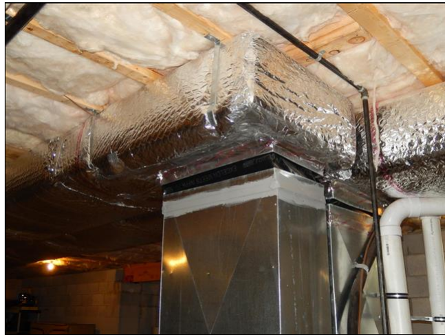
4.3 Item 2(Picture) Return duct
