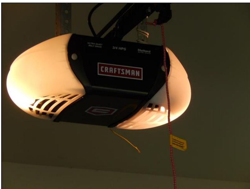
10.0 Item 3(Picture) Garage door opener
