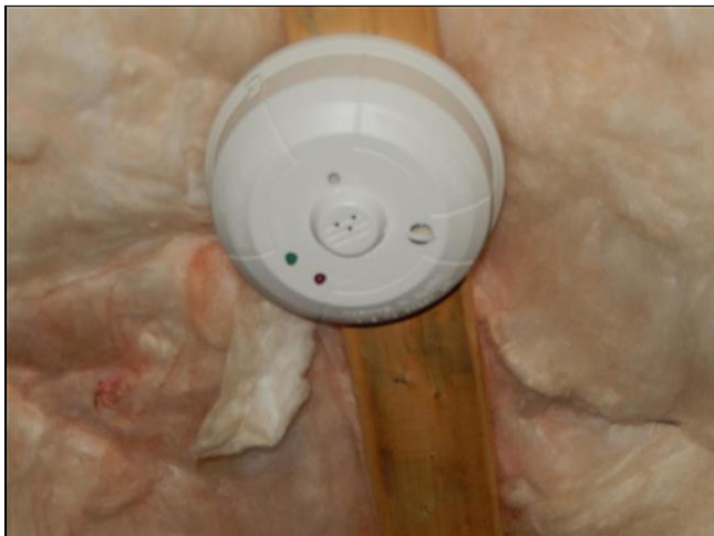
6.7 Item 1(Picture) Basement smoke alarm
