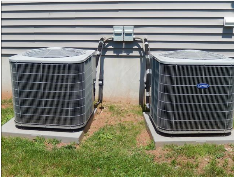
4.6 Item 1(Picture) A/C condensing units
