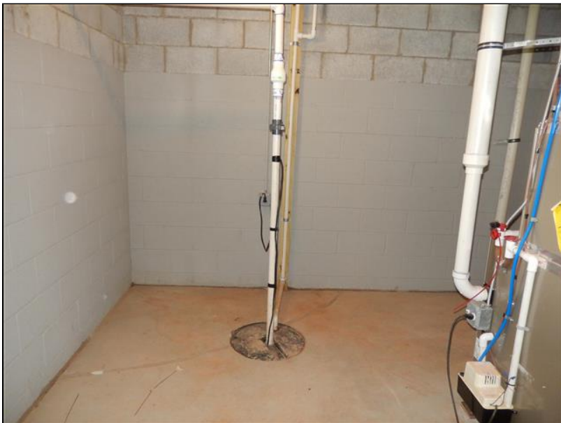
5.6 Item 1(Picture) Sump pump well
