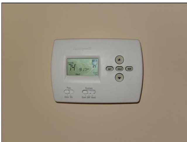
4.1 Item 2(Picture) 2nd floor thermostat
