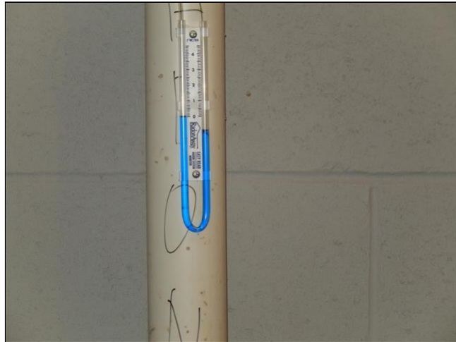
8.3 Item 4(Picture) Manometer
