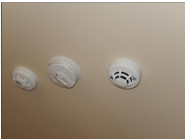
6.7 Item 3(Picture) Smoke, fire and CO alarms, main hall
