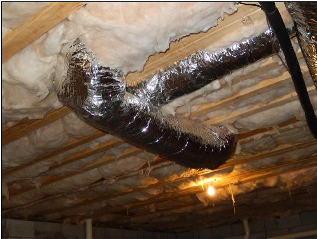
4.3 Item 1(Picture) 1st floor supply duct
