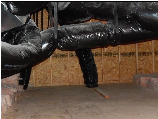
4.3 Item 5(Picture) Insulated duct work
