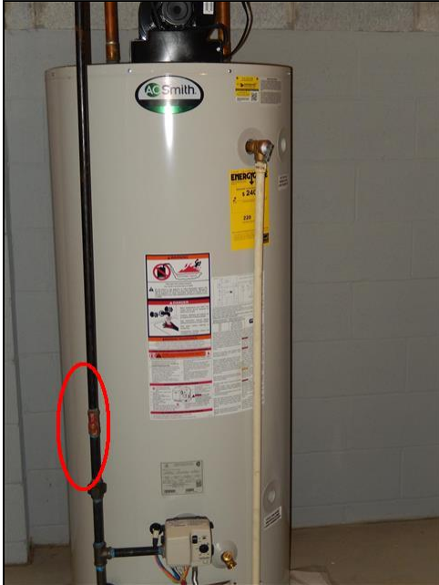
5.2 Item 1(Picture) Water heater
