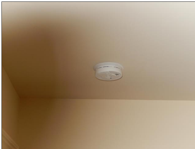
6.7 Item 2(Picture) Smoke alarm, master bed room
