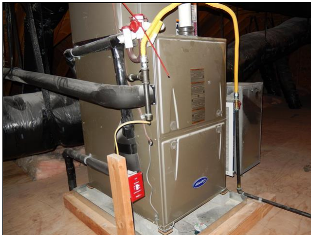
4.0 Item 2(Picture) Upstairs furnace
