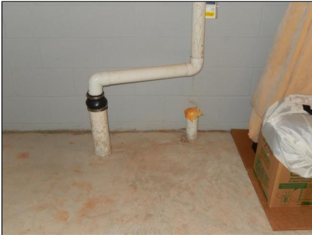
8.3 Item 3(Picture) Radon mitigation piping
