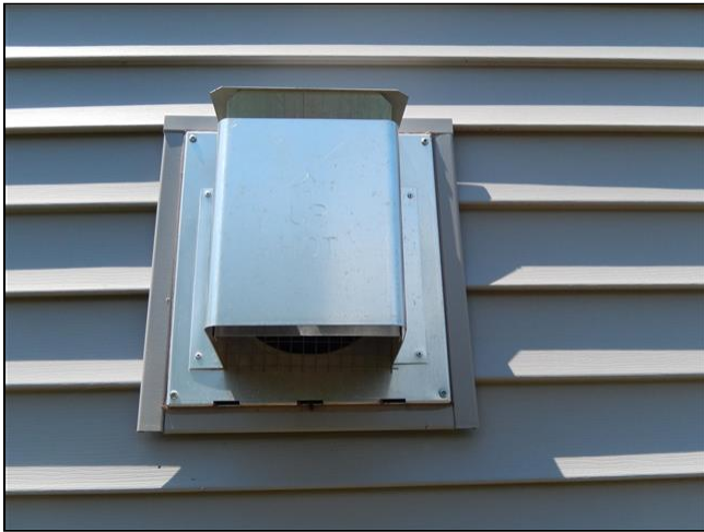
7.2 Item 1(Picture) Fireplace exhaust
