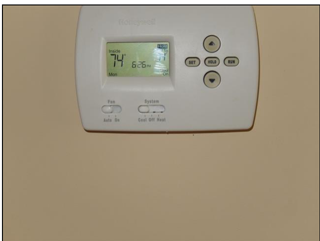
4.1 Item 1(Picture) 1st floor thermostat
