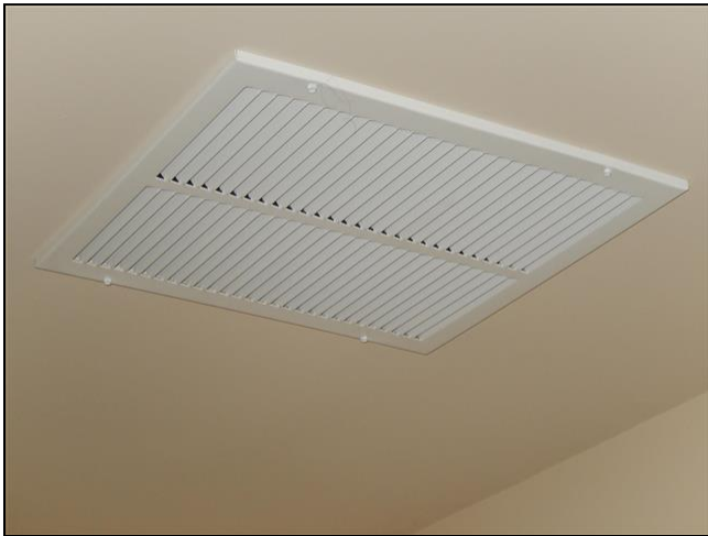
4.8 Item 1(Picture) Return grill - typical
