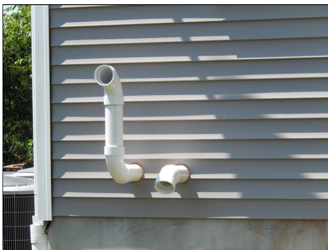
4.5 Item 2(Picture) Lower furnace exhaust and intake
