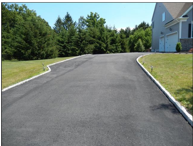
2.2 Item 3(Picture) Driveway seam
