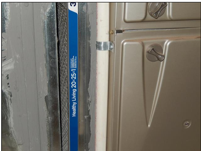
4.3 Item 7(Picture) Downstairs furnace filter
