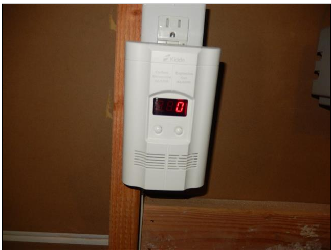
6.8 Item 1(Picture) CO alarm in basement
