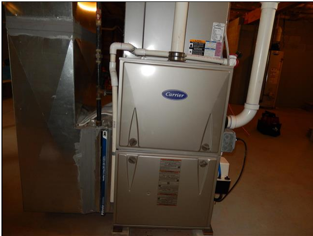
4.6 Item 2(Picture) Lower air handler
