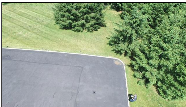
2.2 Item 2(Picture) Driveway corner seam
