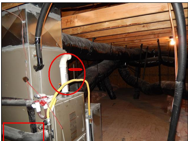
4.5 Item 1(Picture) Upper furnace venting
