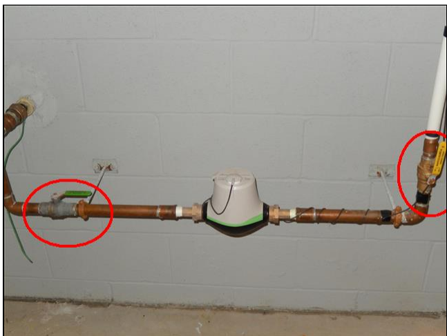
5.0 Item 1(Picture) Water meter
