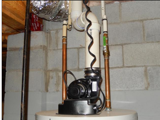
5.2 Item 2(Picture) Water heater venting
