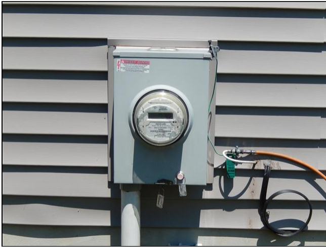
6.1 Item 1(Picture) Electric meter
