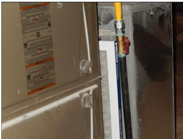
4.3 Item 8(Picture) Upstairs furnace filter
